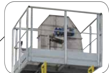
Head inspection platform
