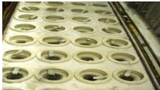
Vac Truck Filter set that have broken filters letting foreign materials into the blower seals and blades
